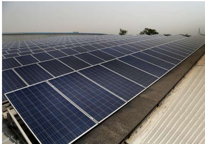
Solar panels at our Faridabad Plant in India
